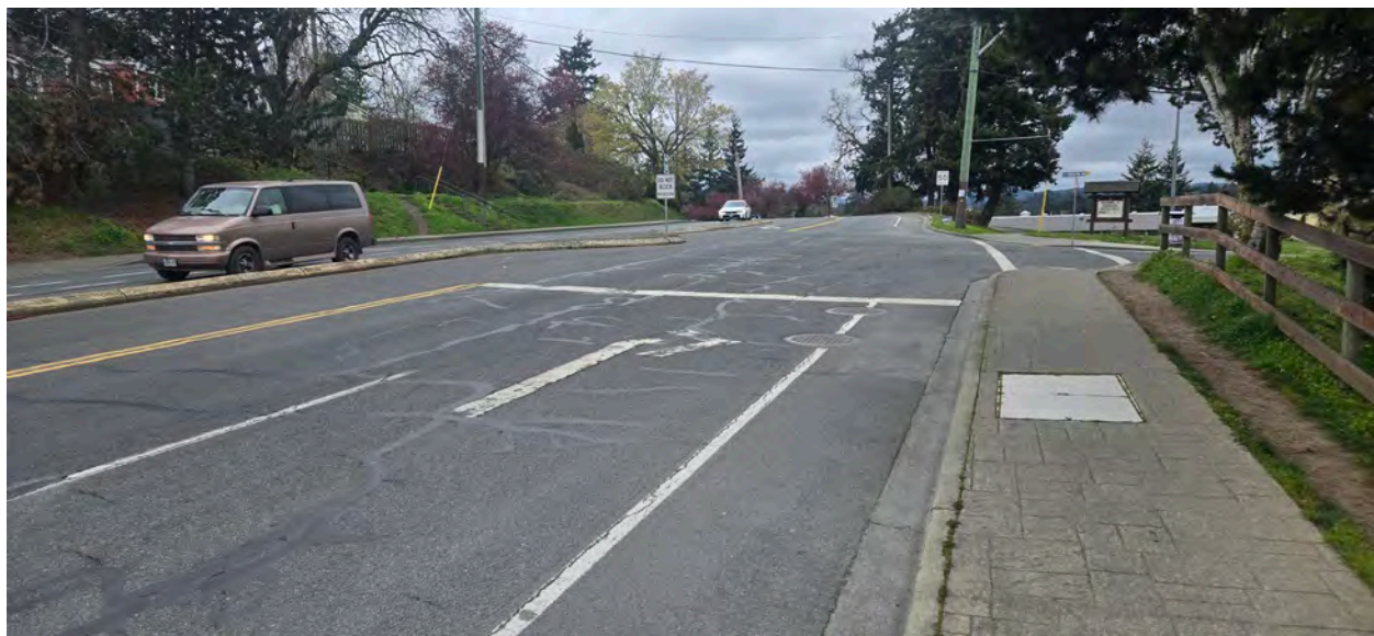
Figure 4.12: Site Visit Photo – Faded Turn Arrow Paint Marking at Island Highway & Shoreline Road
